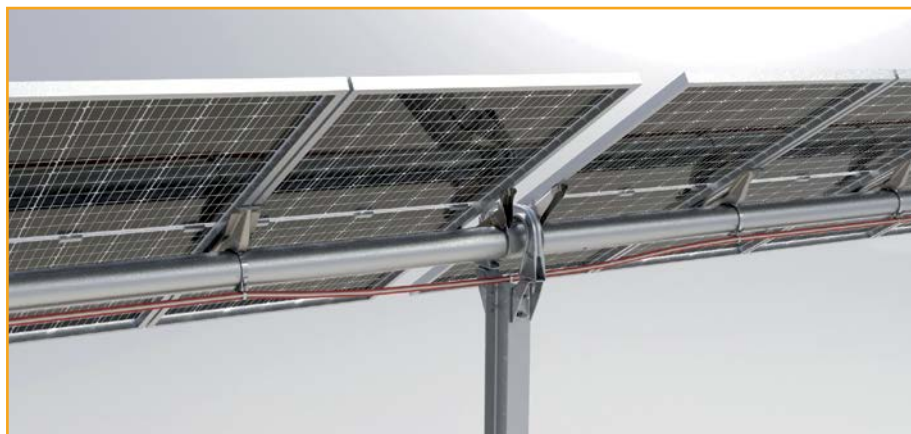
FIGURE D1 For large wire bundles, installers can add wire hangers or harnesses at each short rail location, providing the necessary support at regular intervals along the torque tube. At each foundation and bearing, installers can use a beam clamp or similar to install wire management hardware that secures and protects the wire bundle while allowing for tracker rotation.
