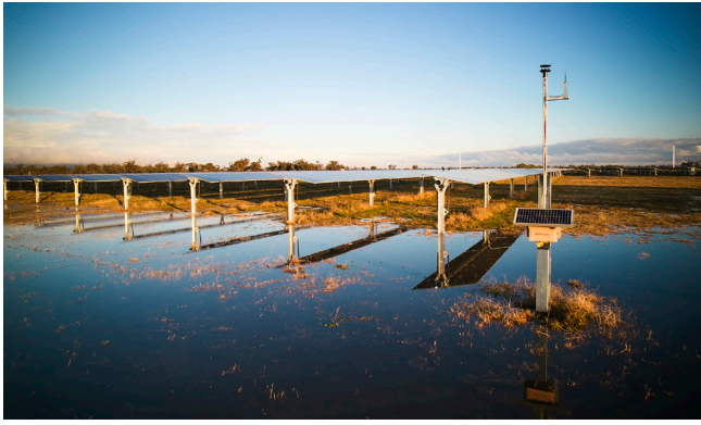
Flooding at Jemalong Solar Farm
